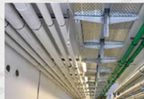
Aqua-Plus Pipes & Aqua-Plus Prins in 5* Hotel compound
